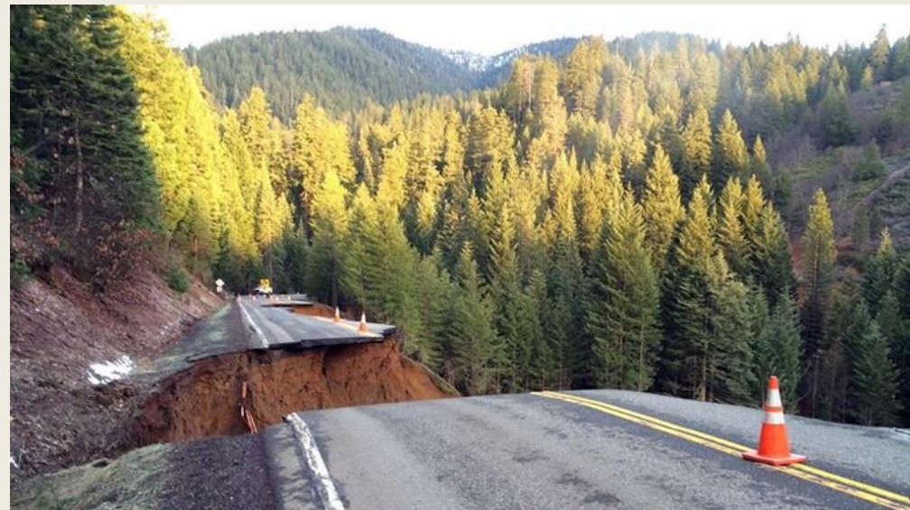
March 16: Northern California highway crumbles as storm-soaked hillside collapses. Highway 3 near Rush Creek Road just north of Weaverville in Trinity County. Photo: LA Times
