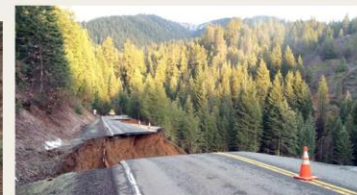
March 16: Northern California highway crumbles as storm-soaked hillsides collapse. Highway 3 near Rush Creek Road just north of Weaverville in Trinity County. Photo: LA Times
