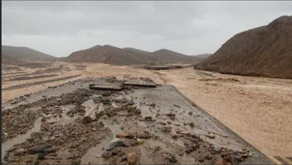
Flooding in Death Valley, NP
